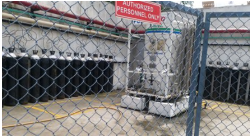
Fig. 1.1 Typical LOX and Compressed O 2 Cylinder system in a large hospital setup
